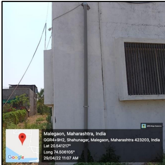
Rainwater Collection Pipe
