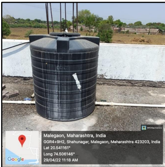
Overhead PVC water storage tank
