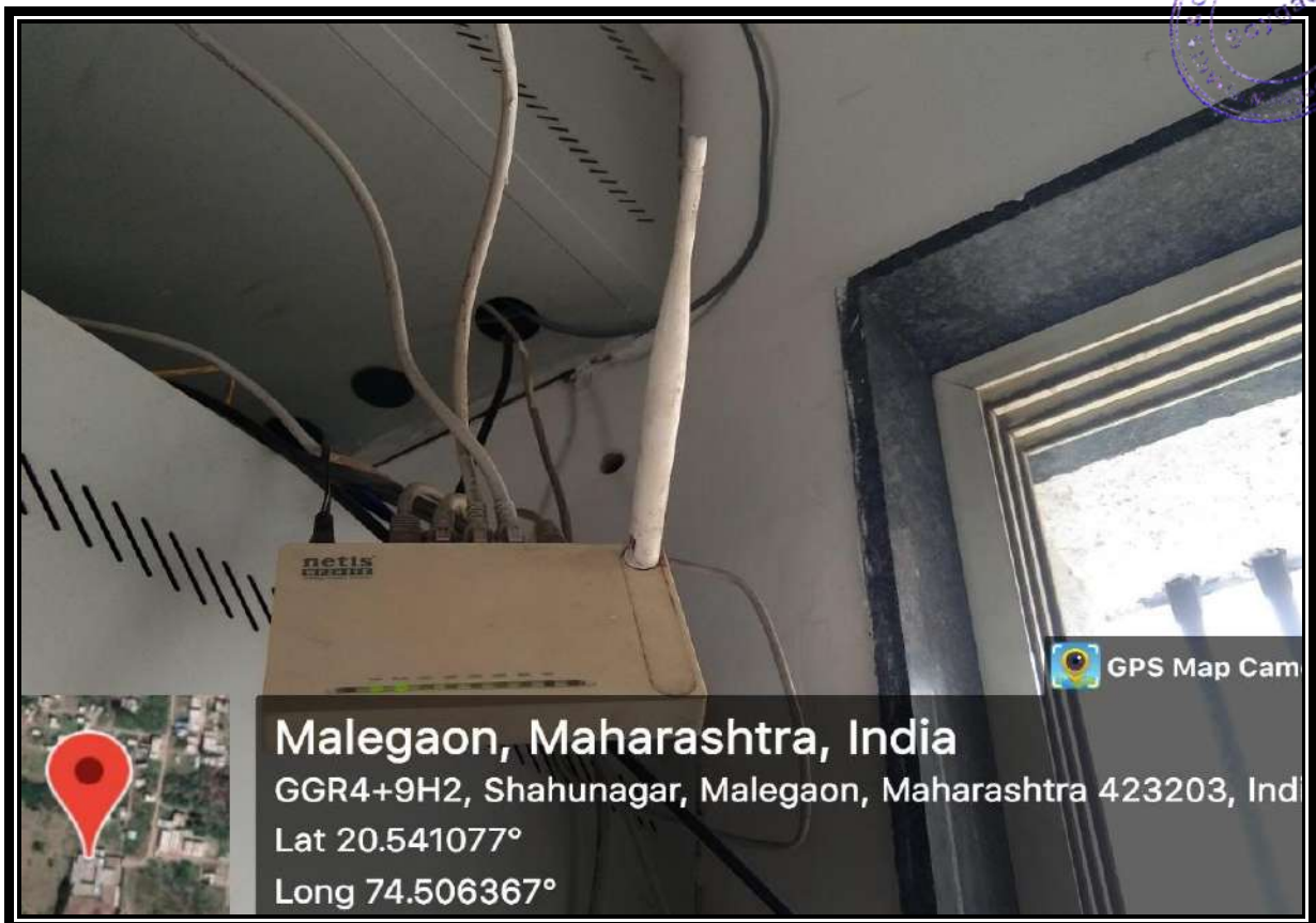
Main Wi-Fi Router
