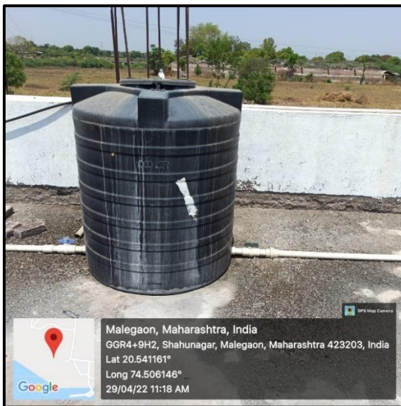
Overhead PVC water storage tank
