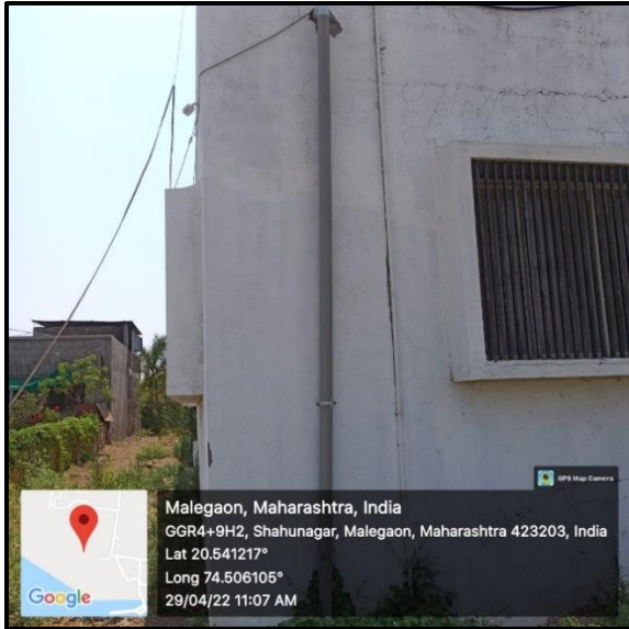
Rainwater Collection Pipe
