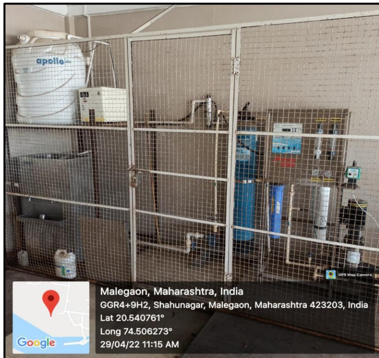
RO system installed in the college for drinking water
